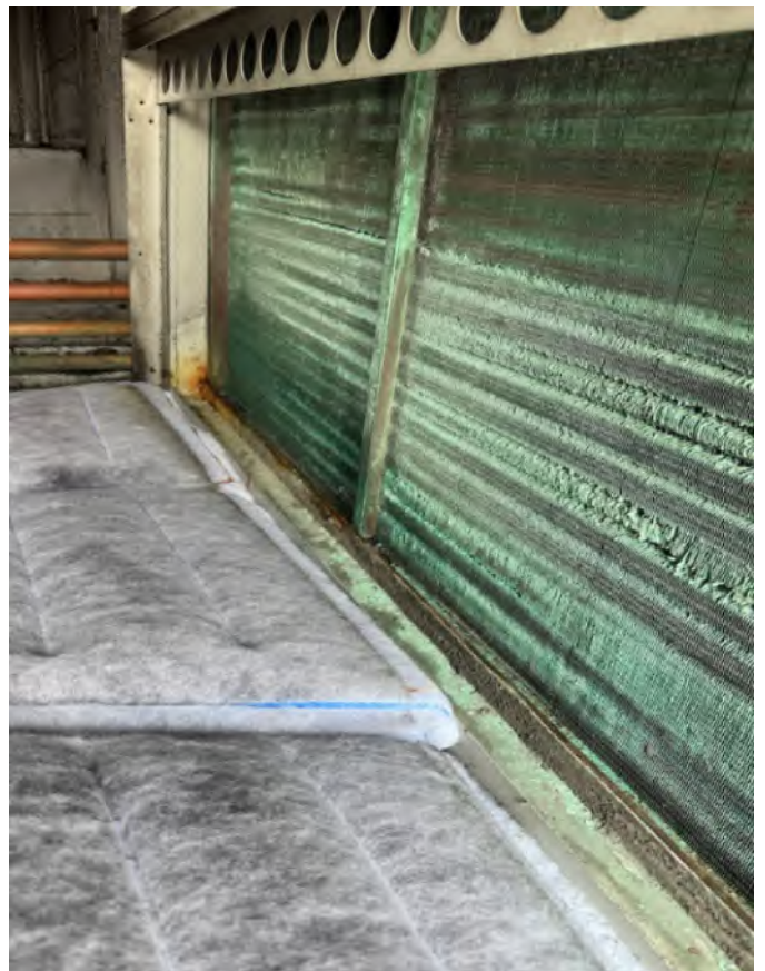
Interior Coils Green Corrosion / Oxidation on HVAC Coils caused by moisture
