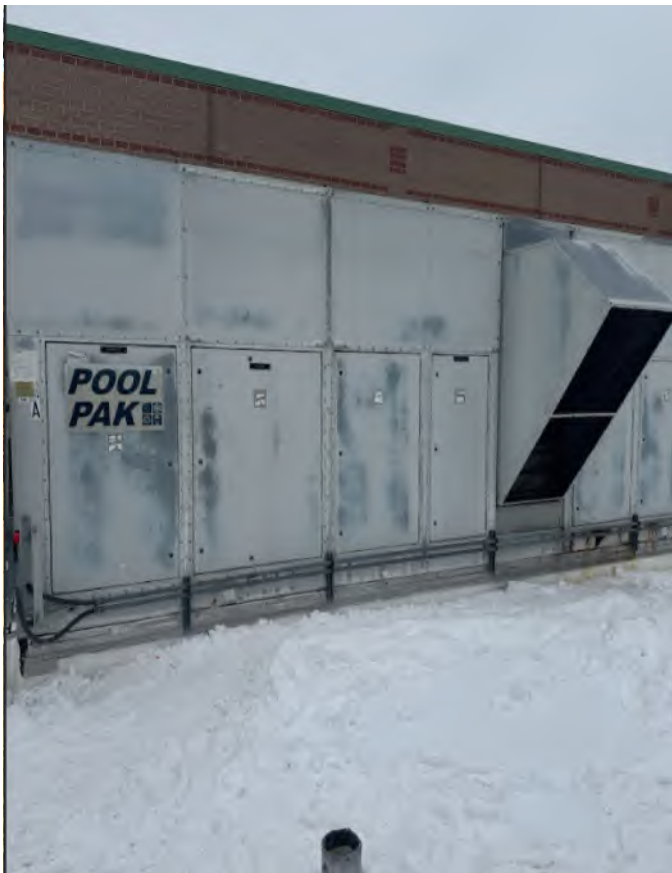
Exterior of PoolPak Unit Roof top unit
