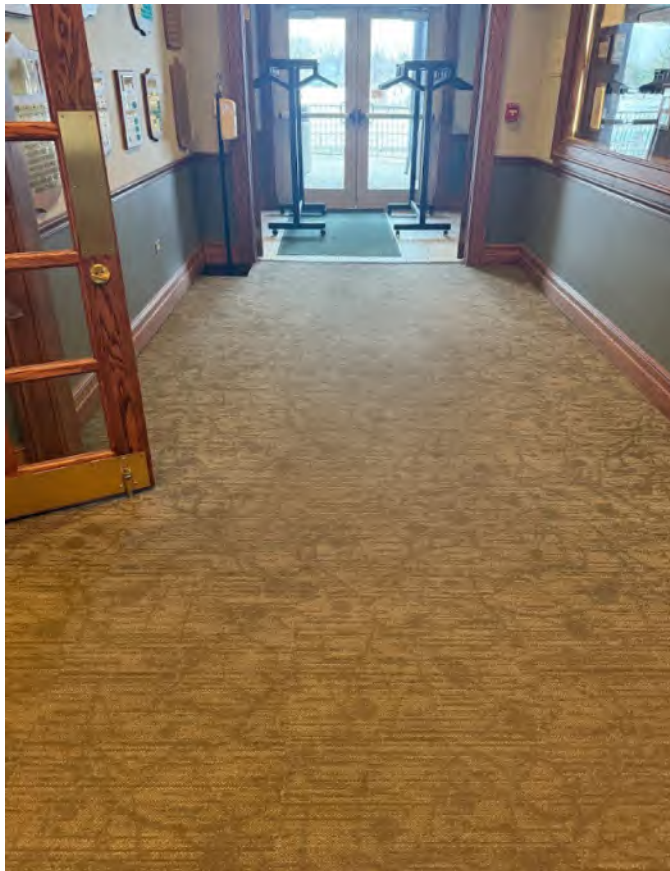
Hallway / Lobby Wear pattern down center of corridor
