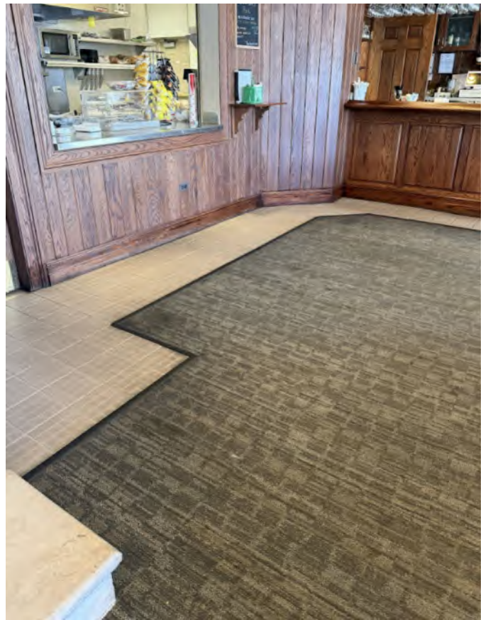
Bar / Grille Area Heavy wear at pickup window and staining at entrance to kitchen
