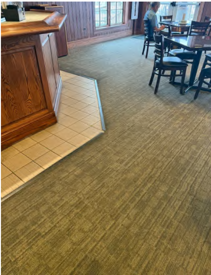
Bar / Grille Area Heavy wear in front of bar
