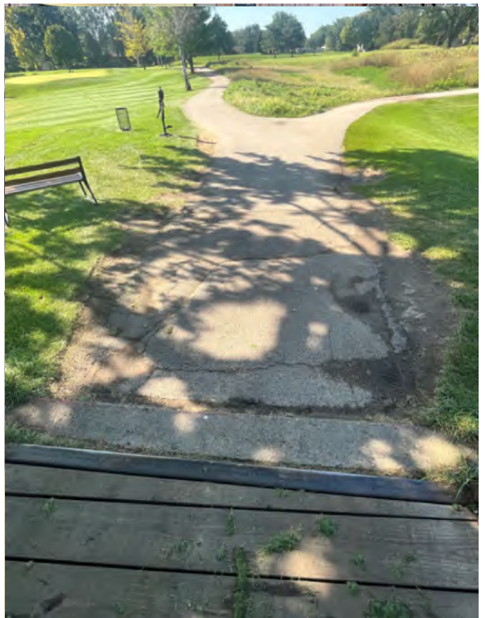
Hole 10 Over the bridge - Asphalt sags at bridge entry and cracking
