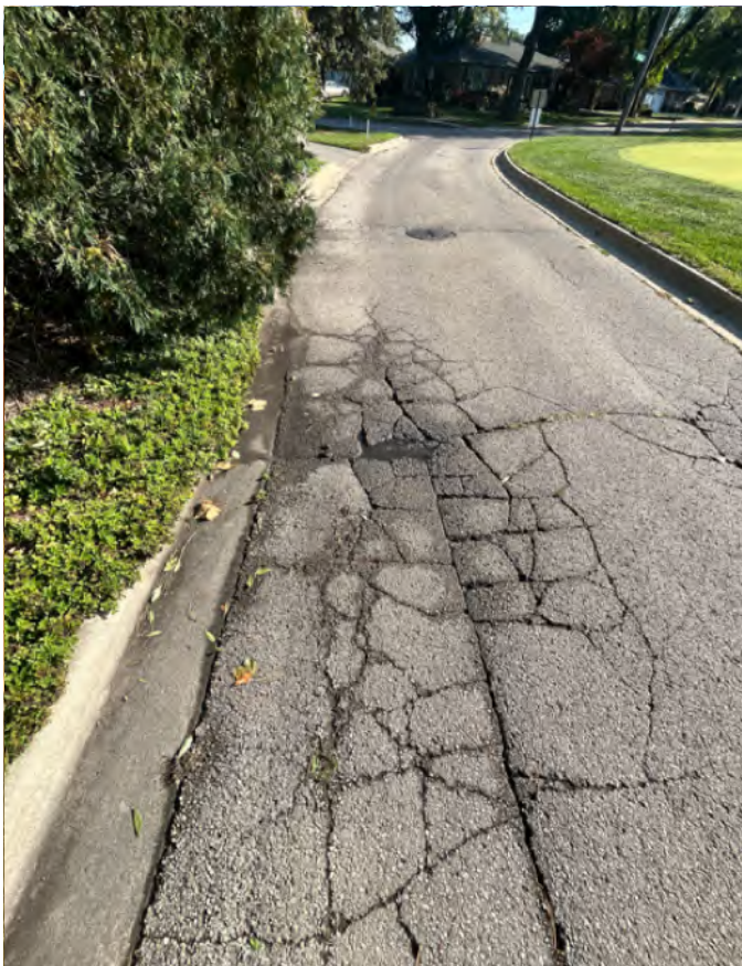
Service Drive Cracking and holes in asphalt drive
