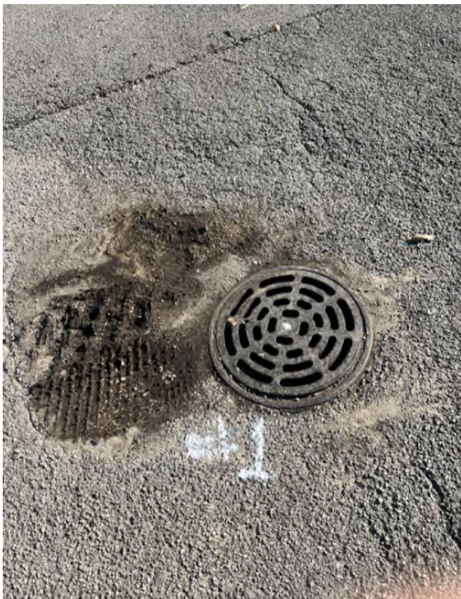
Manhole Adjustment Asphalt around manhole degrading
