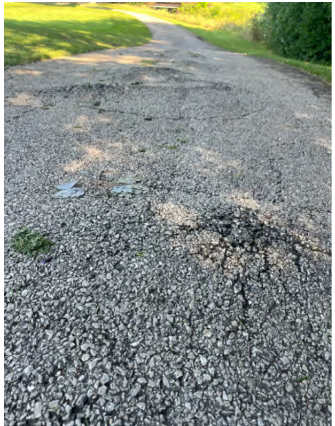
Hole 17 Heaving and buckling asphalt pathway along hole
