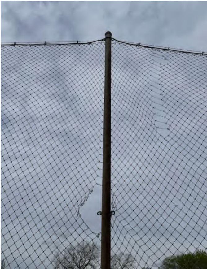
Holes in netting system field 1
