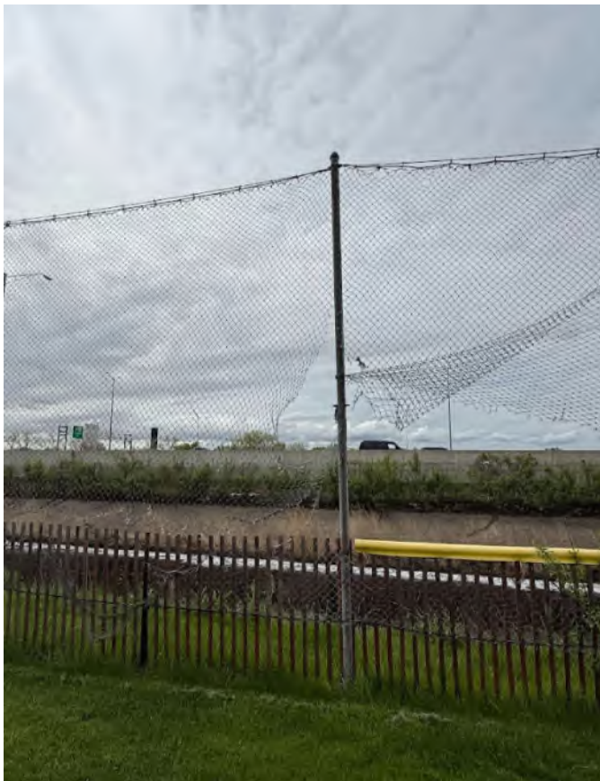
Holes in netting system field 2
