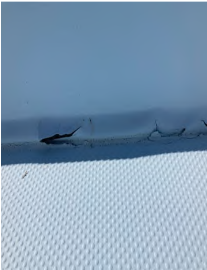
Existing Liner Cracking
