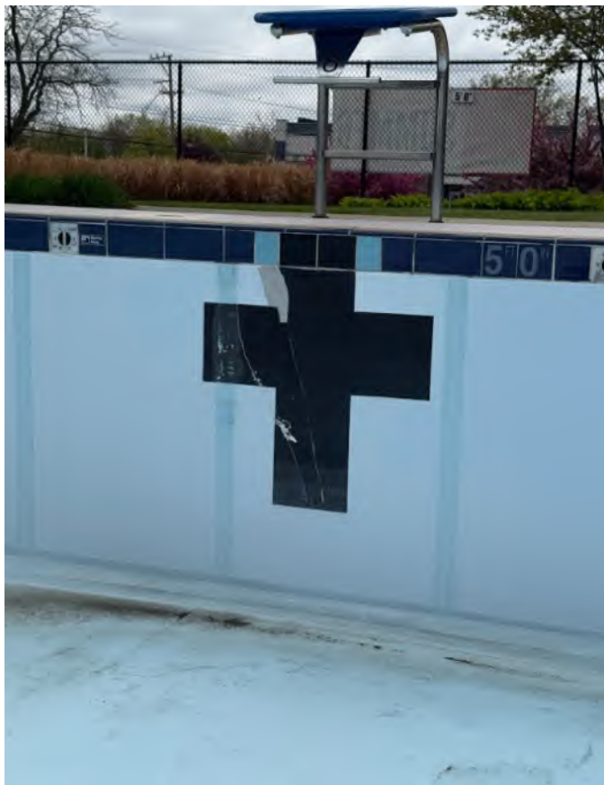
Existing liner cracking off metal wall
