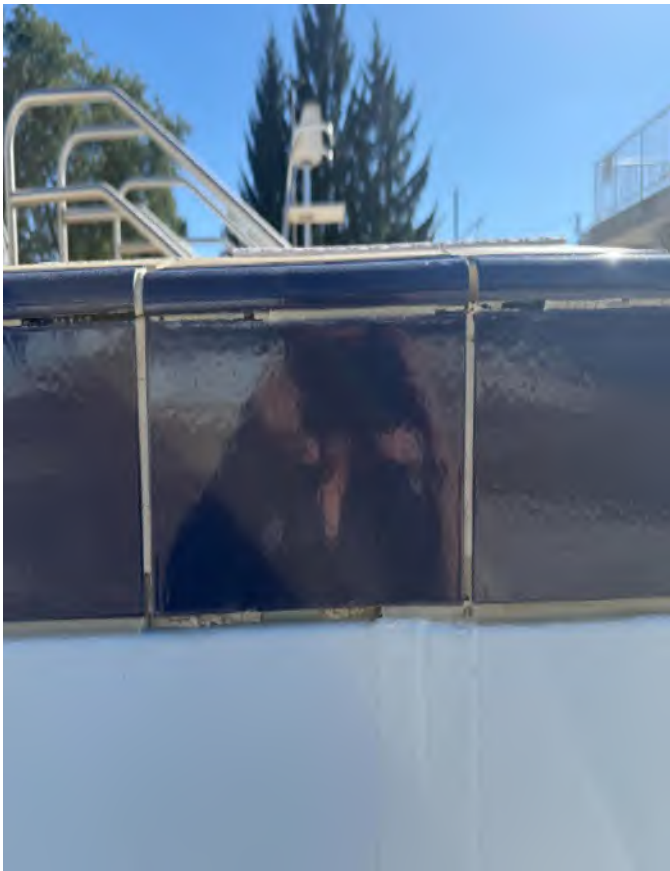
Current failing grout and silicone
