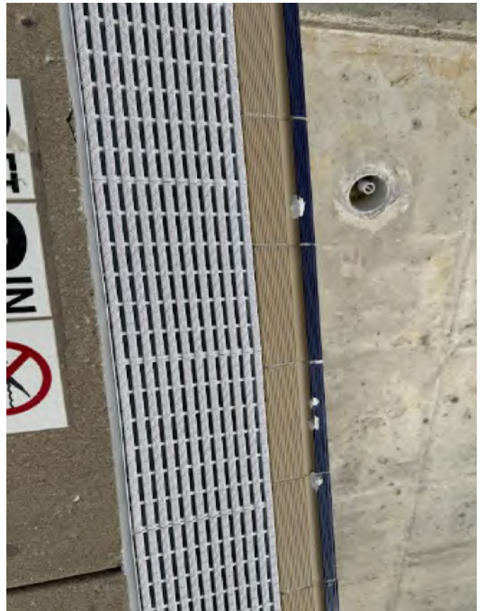
White patched areas at handhold tile
