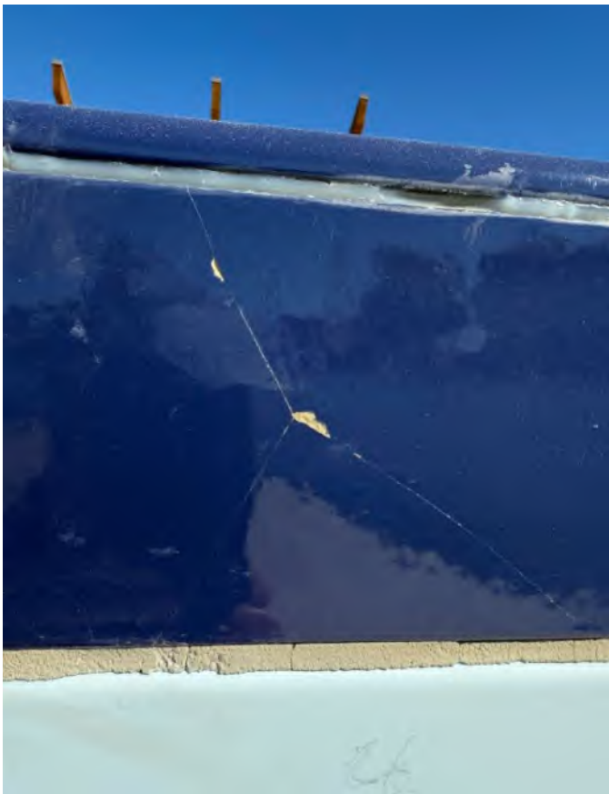
Cracked waterline tile
