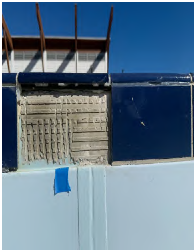
Waterline tile that popped off after silicone removed
